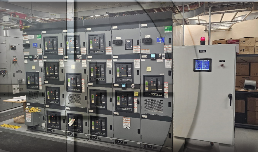
The Naples WRF Generator Control Panel & Operator Terminal.
