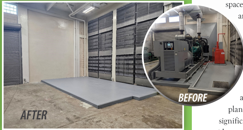
Moving the generators outside allowed for the repurposing of existing generator rooms into an electrical room annex and other future uses.
