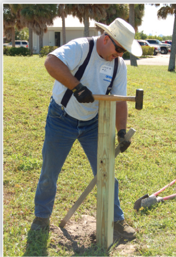
Lonnie helped build a split rail fence as part of the company's 9 th annual Coastal Clean Up at Lover's Key/Carl E. Johnson State Park.
