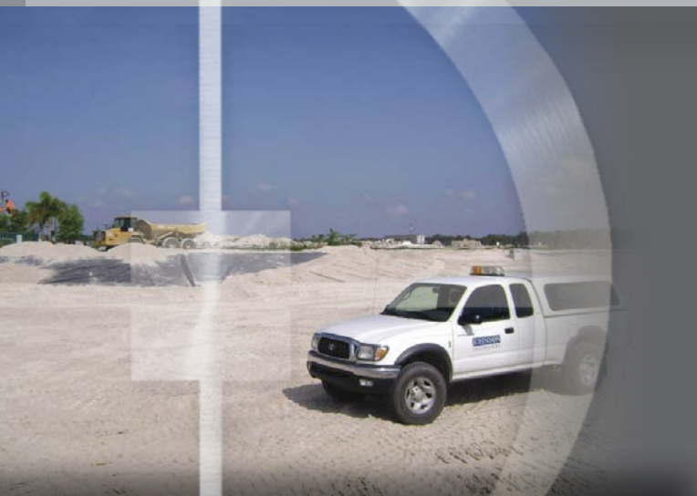
The lake will store 1.5 million gallons of highly treated wastewater to reuse for golf course irrigation.
