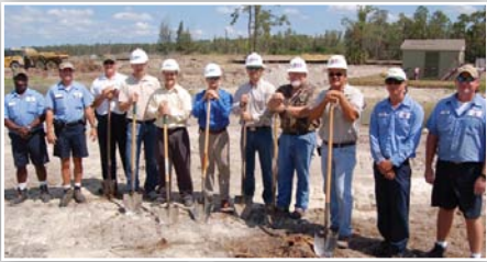
The project groundbreaking at Eastwood Golf Course included Johnson Engineering's key project team Jeffrey Roman, P.E., LEED AP, David Trouteaud and Erik Howard, P.E., along with General Contractor, EHC Inc. and City of Fort Myers staff.
